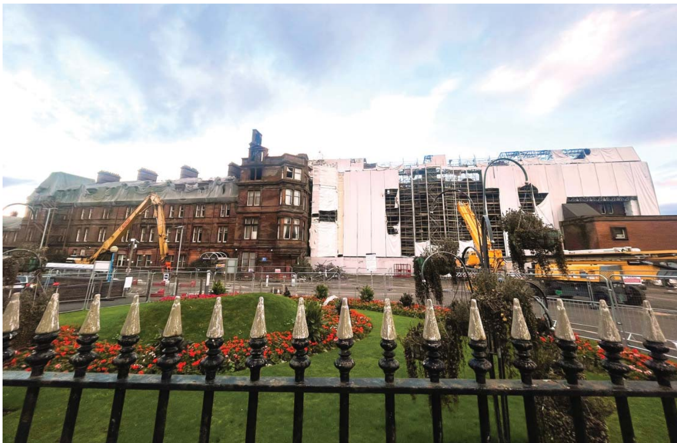
The station hotel post fire, with safety works underway in late October 2023. The south wing is to the right, still largely shrouded in the original scaffolding encapsulation, much of which survived intact from the fire (Credit: © SAVE Britain's Heritage)
