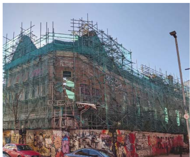
Somehow still standing today, the Garfield Buildings (c.1895-1896) on 2-14 Lower Garfield Street and 56-60 North Street, Belfast City Centre. Credit: Howard Franklin.
