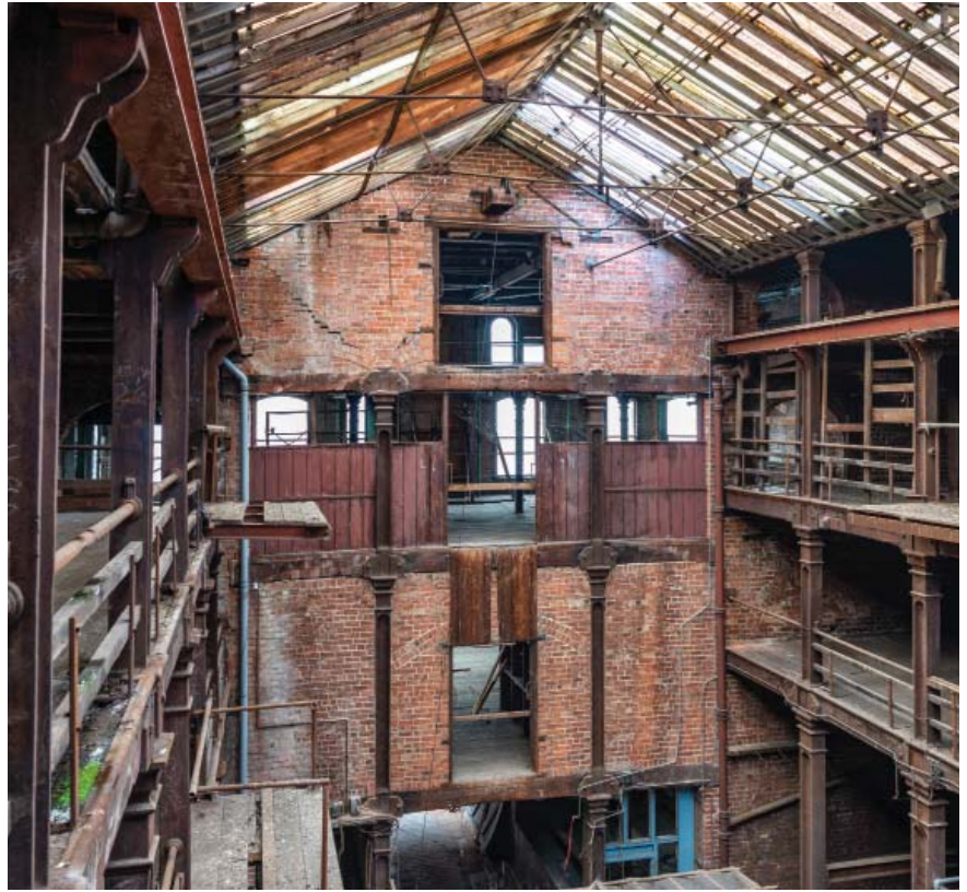
Interior of Riddell's Warehouse. The Hearth Historic Buildings Trust plans to sensitively transform this rare survival into a creative hub with performance space, exhibitions, café and co-working. (Credit: Gary Quigg Photography)
