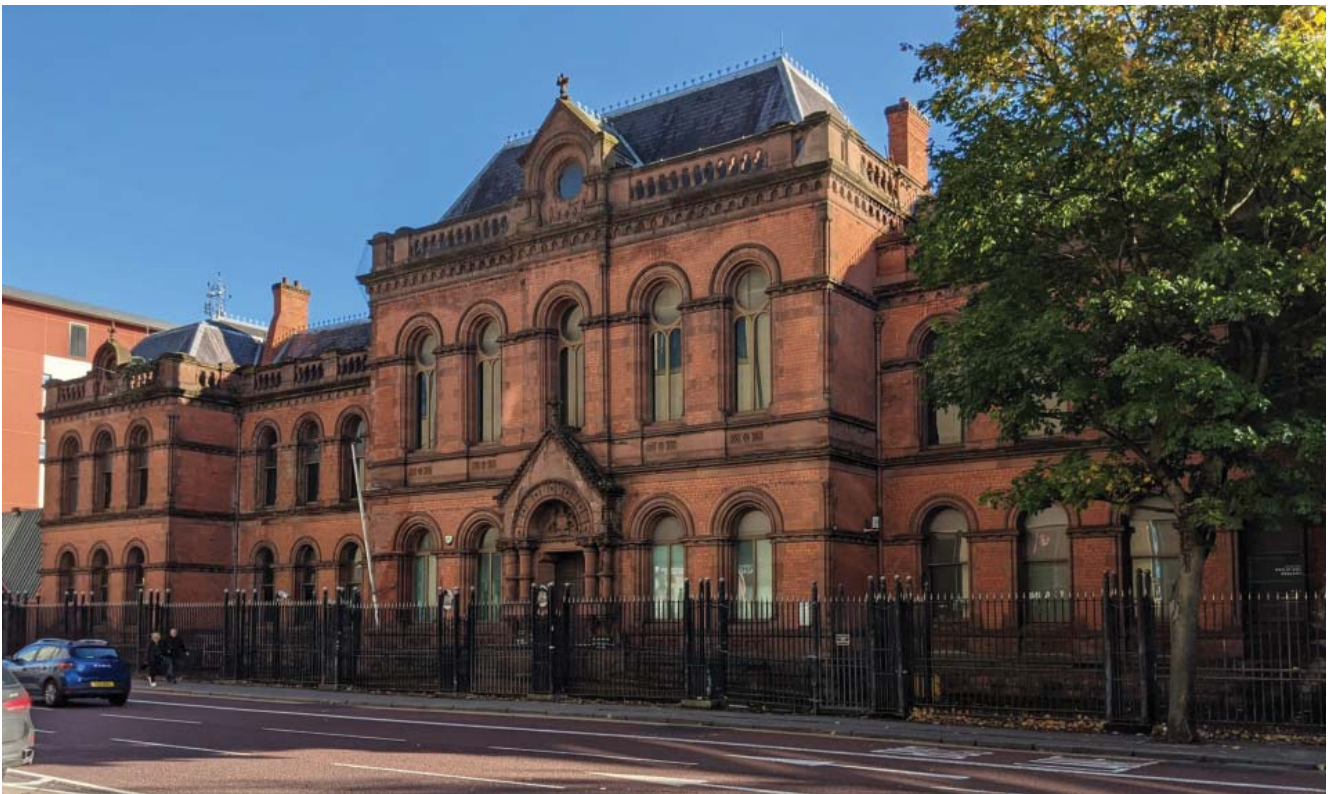
The Old Town Hall in Belfast City Centre (c.1869-71), currently vacant and deteriorating. (Credit: Howard Franklin)
