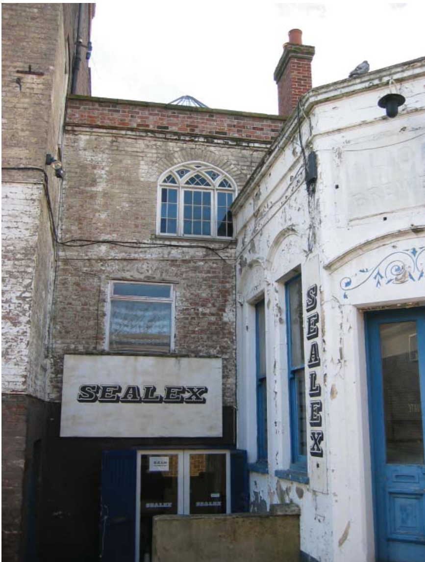
Rear section of Chatham House adjoining brewery buildings, March 2007. (Credit: Medway Council)
